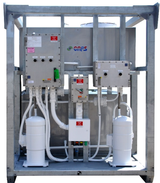
Electrical Panel View NEMA 7 Explosion Proof Stainless Steel Cabinet & Hot Dipped Galvanized Skid & Cage
