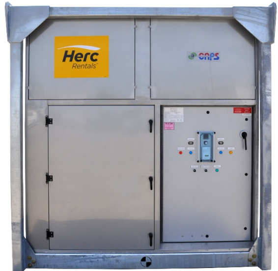
Control Panel View
